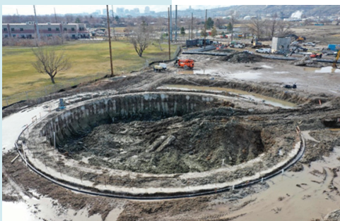
Influent Pump Station
